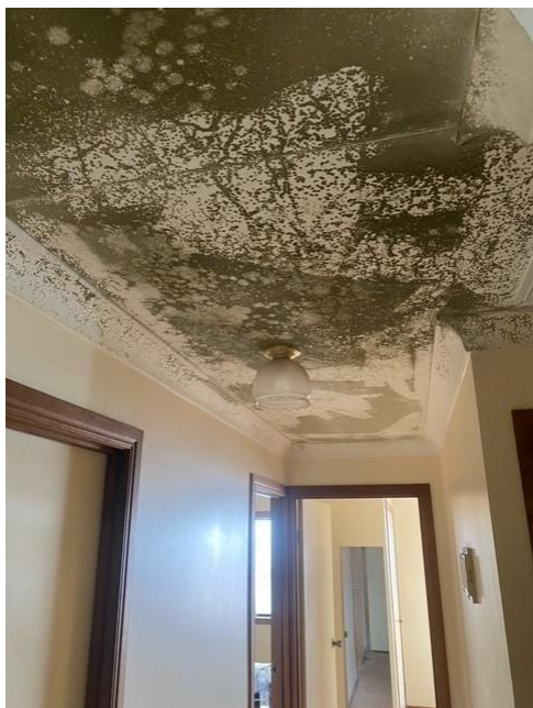
Ceiling Mould – Toowoomba
